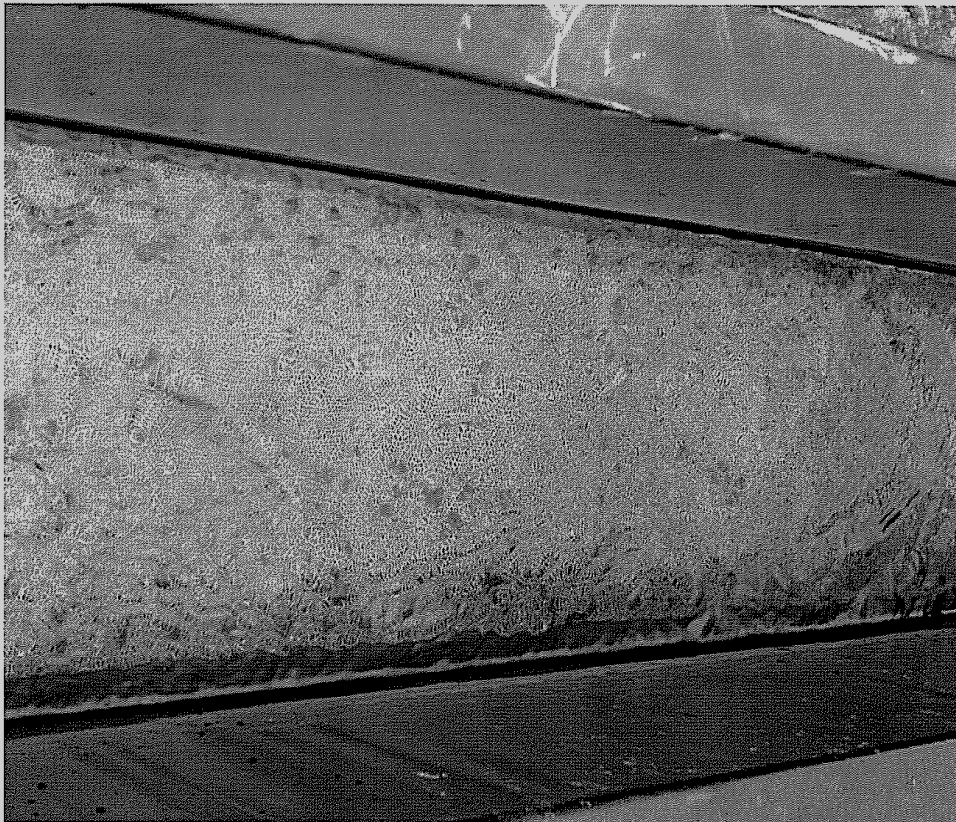
Image 2, fouling on the screens
