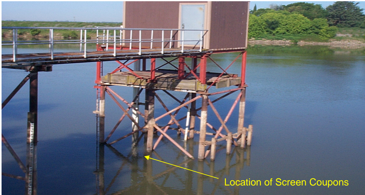
Figure 3. Hood Monitoring Station RSAC 142 and location of screen coupons.
